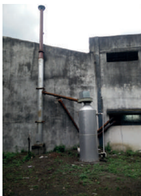
CENTRALIZED SCRUBBER SYSTEM
